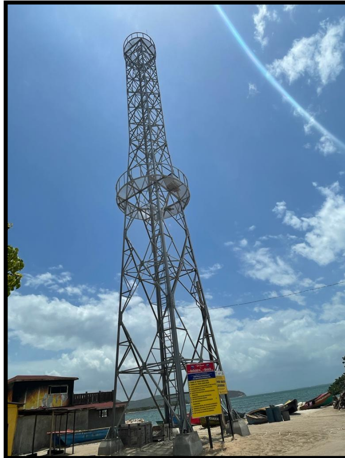
30 meter lattice steel tower
