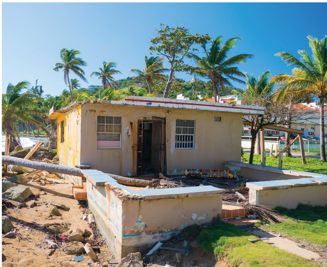
Figure 16. Catastrophic erosion and infrastructure damage in Puerto Rico due to Hurricane María
