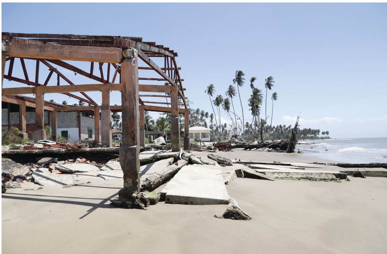
Figure 13. Displacement towards land of the active escarpment as clear evidence of the erosive tendency of a beach. Granville, Cedros, Trinidad
